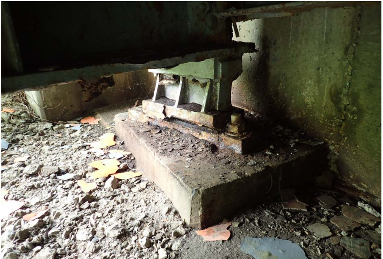
Upstream abutment 1 bearing; flaking paint with moderate corrosion.
