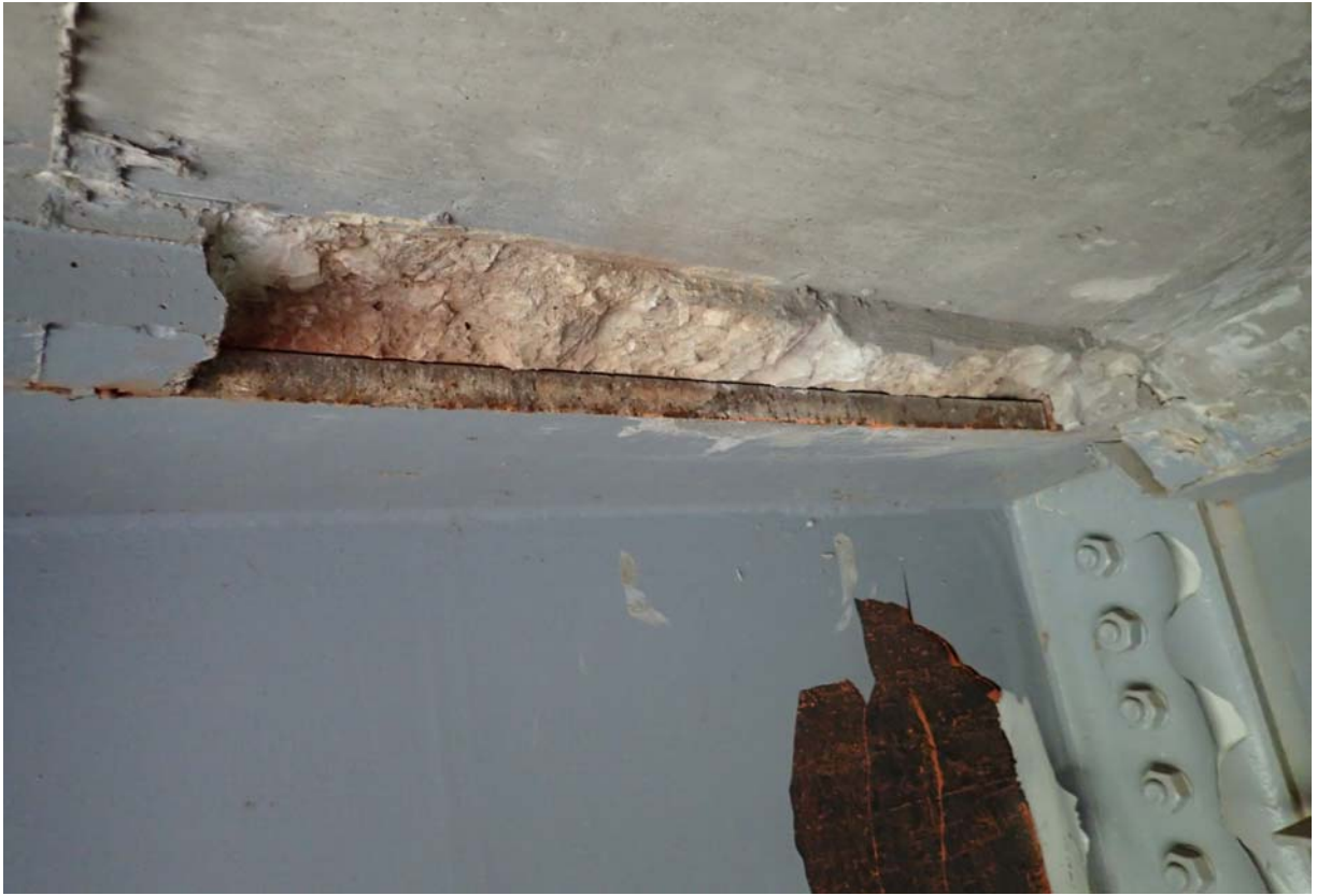
View of spalling along the fillet above girder 2 from upstream at abutment 4.
