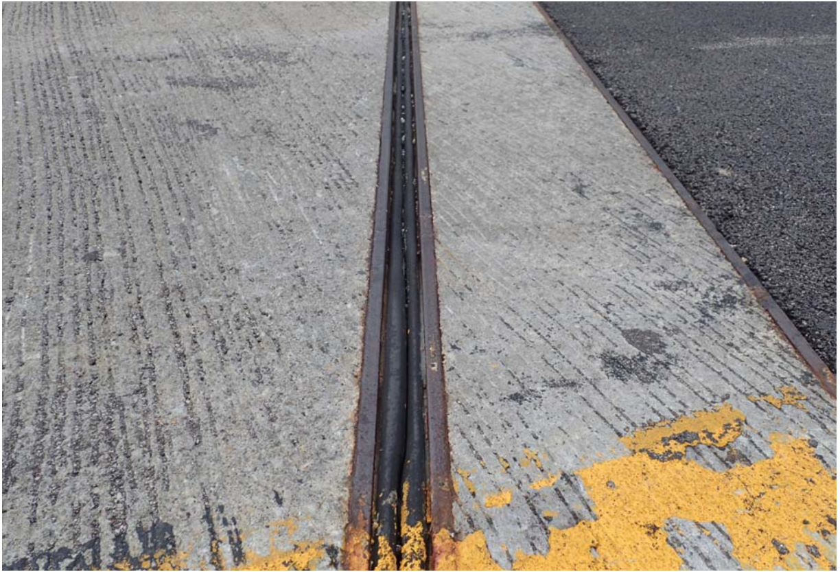
View of the transverse joint at abutment 1. It is impacted with minor debris and has some adhesion failure.
