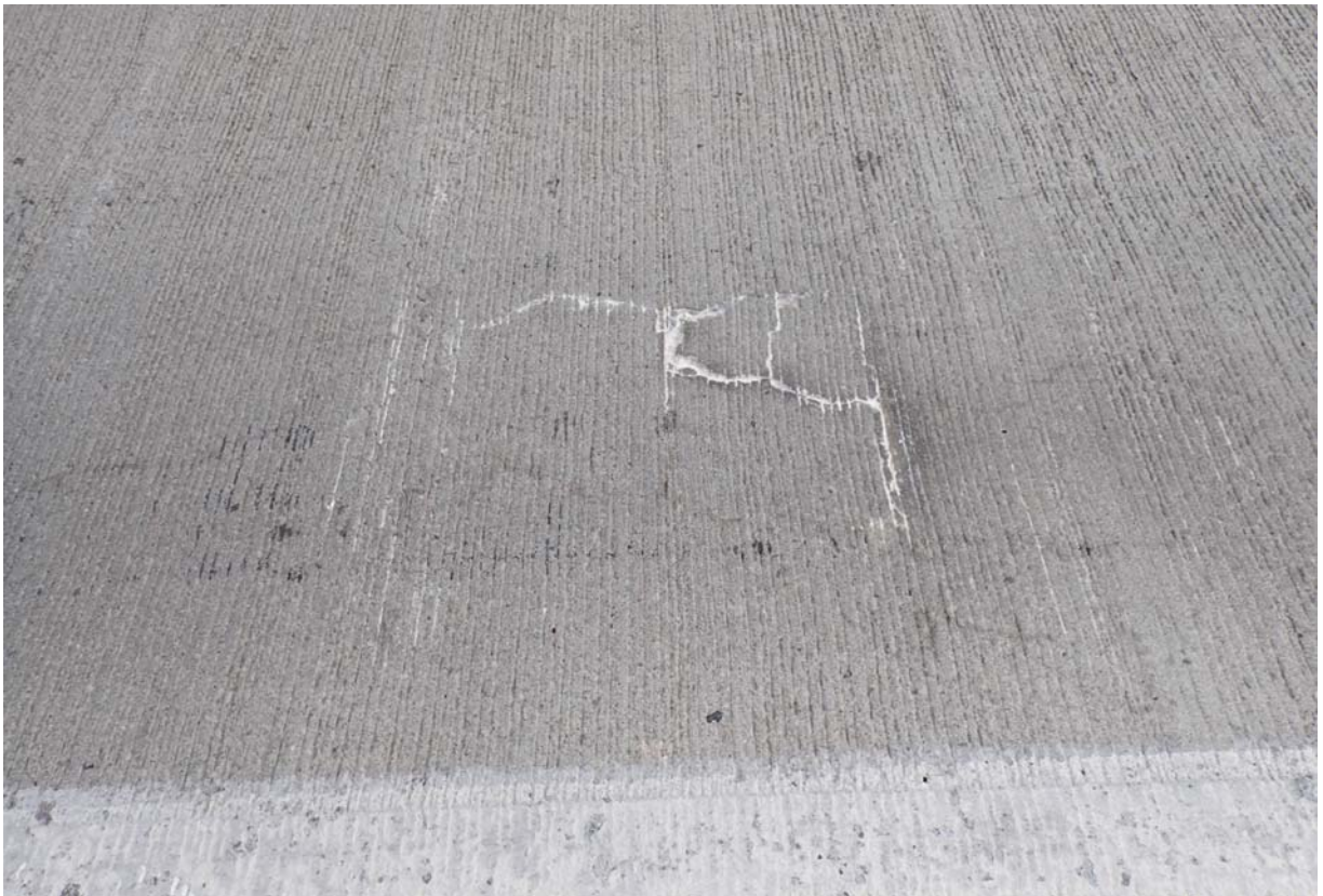
View of an area of moderate cracking with efflorescence in the wearing surface of the slow lane in span 1.
