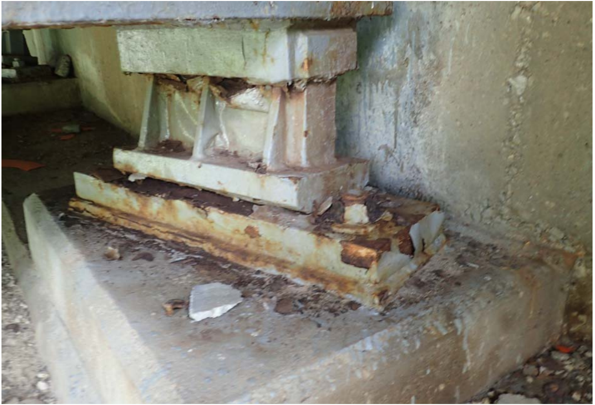
Upstream bearing at abutment 4; flaking paint with some moderate corrosion.
