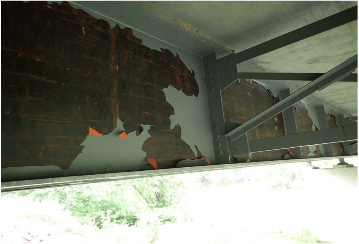
View of widespread paint failure on the downstream face of girder 3 in span 3.
