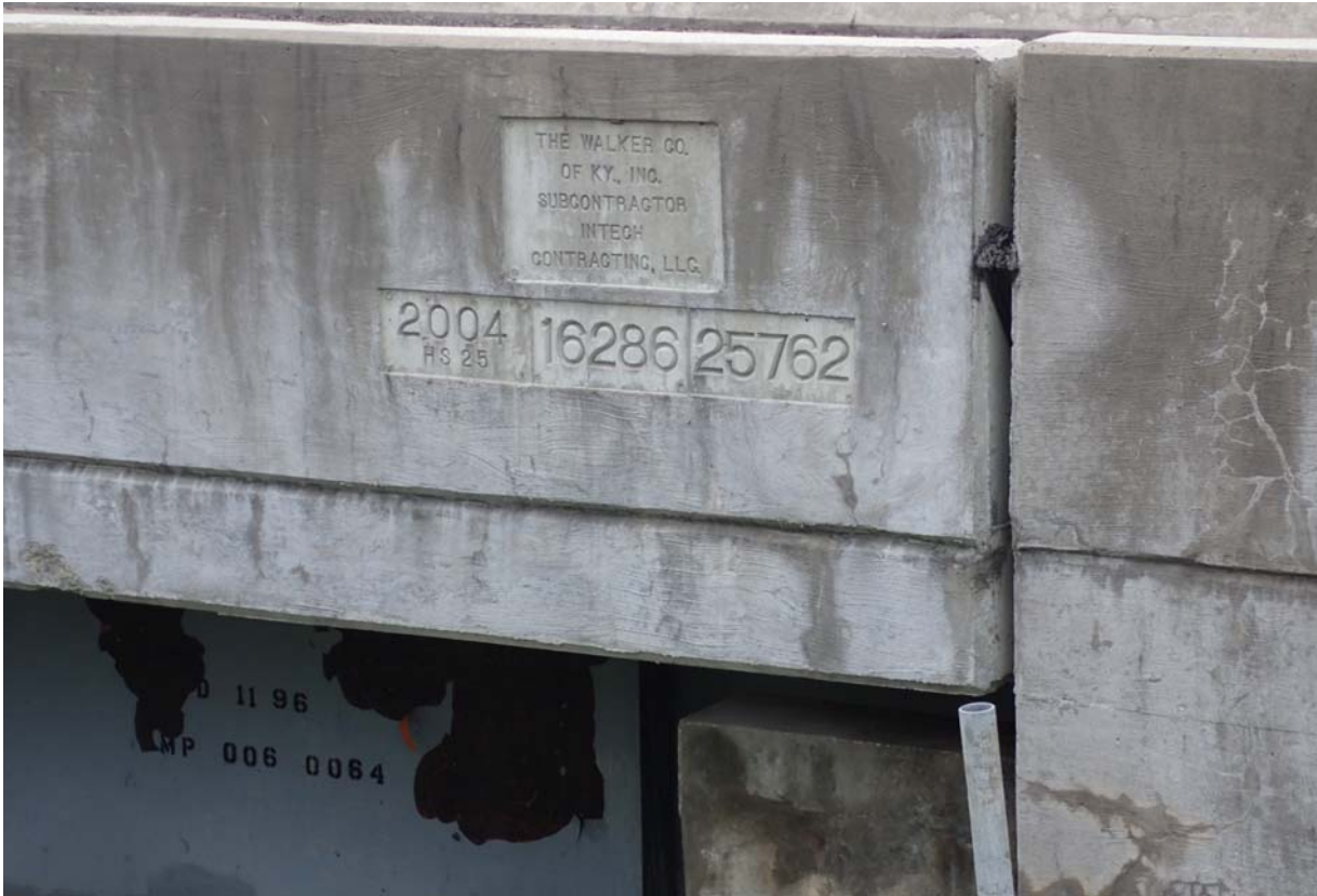
View of the stamps on the downstream face of the barrier/beam at abutment 1.
