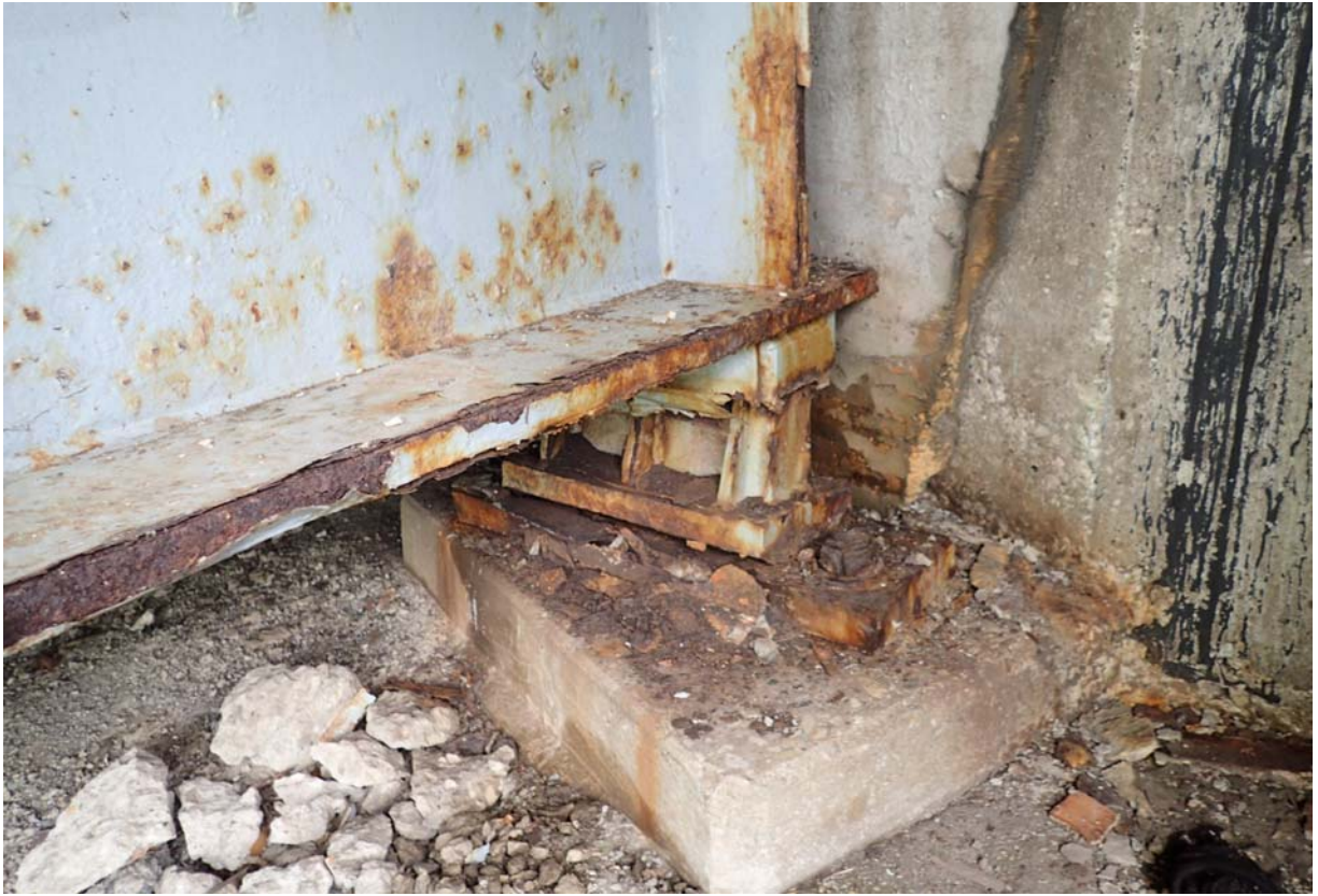
Downstream abutment 1 bearing; flaking paint with moderate corrosion. Notice the flaking paint along the girders bottom flange and the exposed steel has moderate rusty corrosion.
