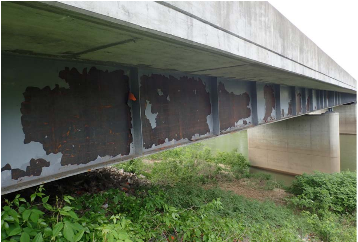
View of widespread paint failure on the exterior face of the downstream girder in span 3.
