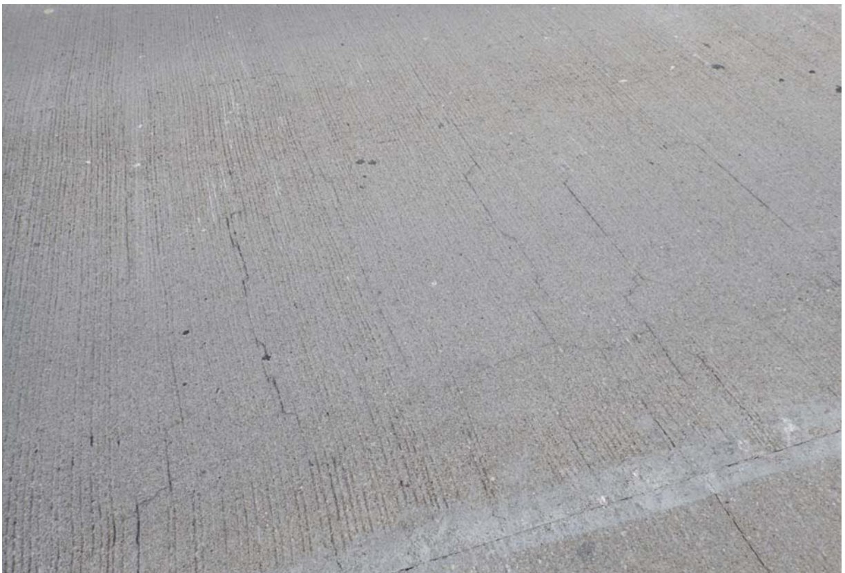
View of several minor sized transverse cracks in the wearing surface of the slow lane
