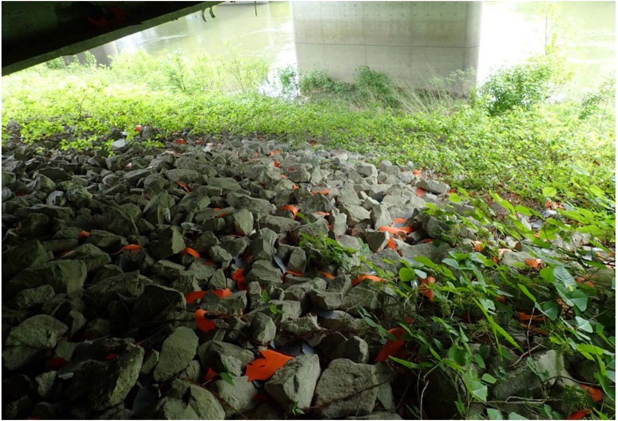
Paint scattered across the ground in span 1.
