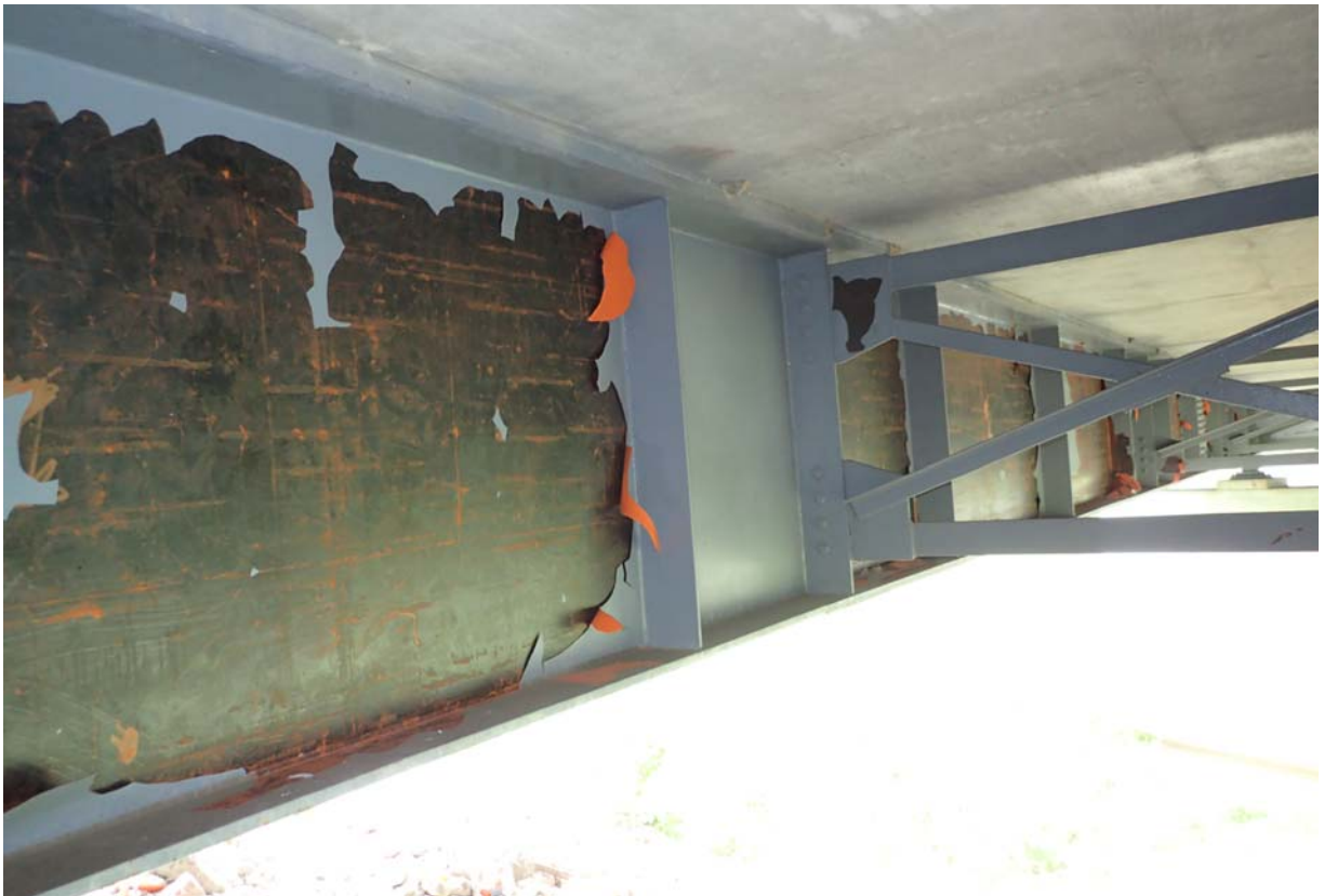
View of widespread paint failure on the downstream face of girder 2 in span 3.
