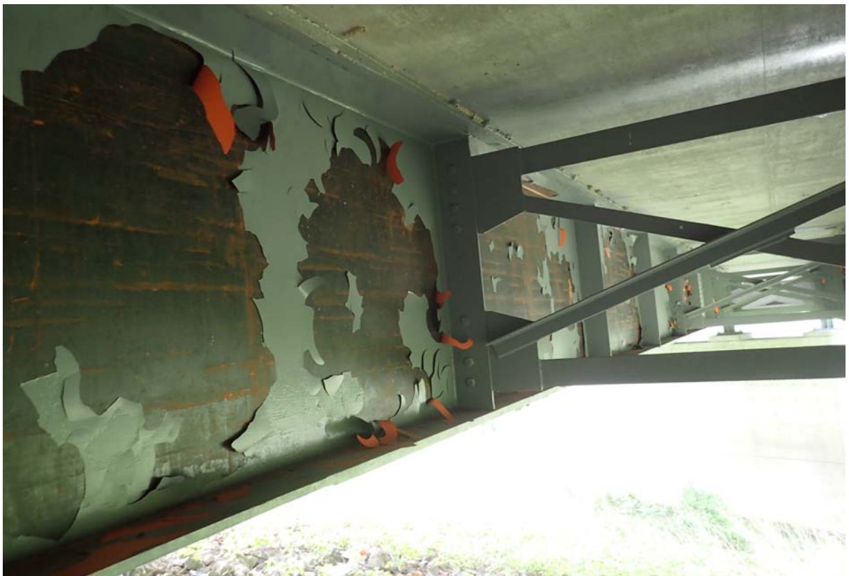
Several large areas of paint failure on the upstream face of girder 2 from upstream near abutment 1.
