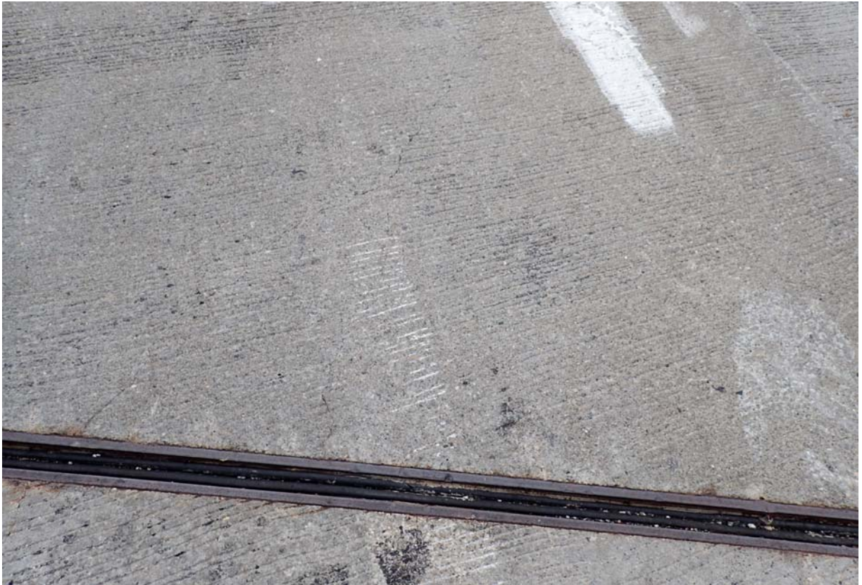
View of some minor sized diagonal cracking in the wearing surface near abutment 1.
