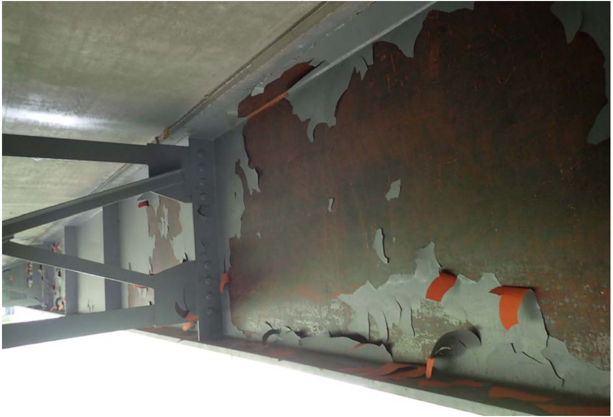
Several large areas of paint failure on the downstream face of the upstream girder near abutment 1.
