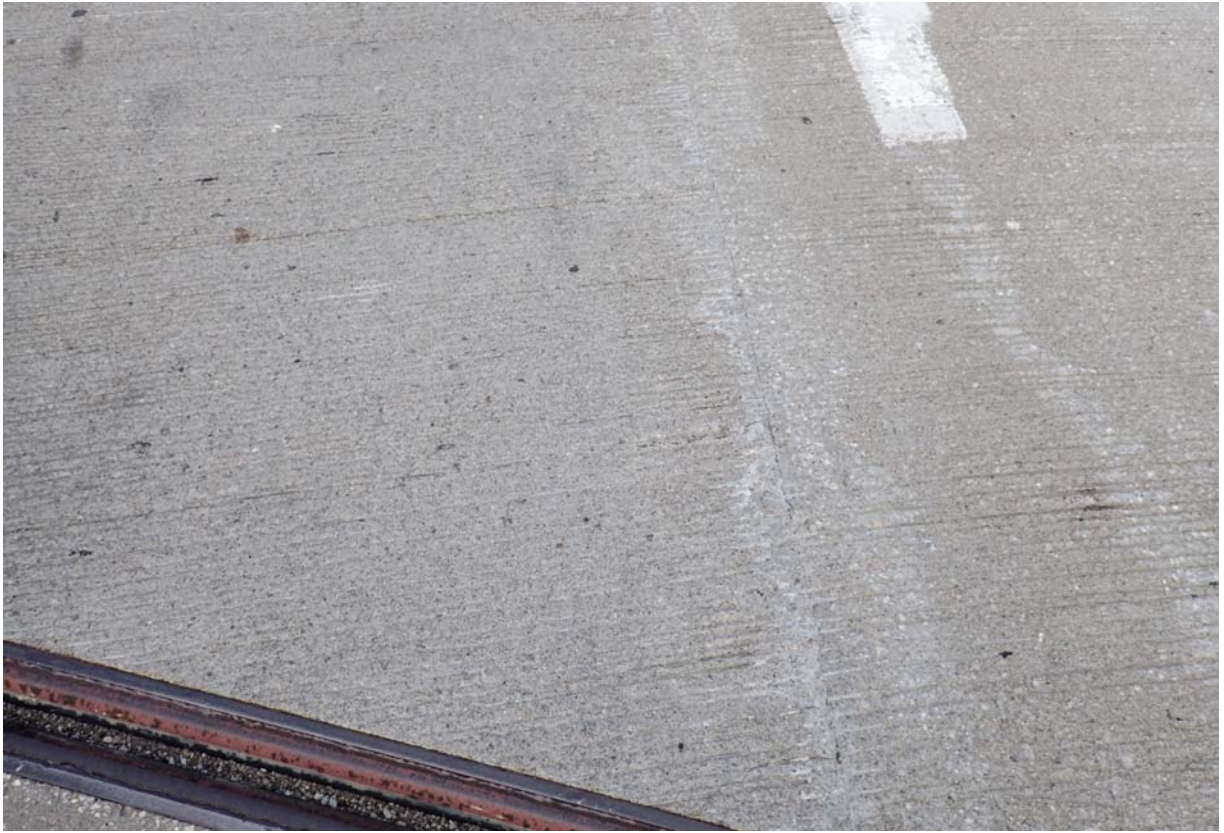
View of minor sized longitudinal cracking in the wearing surface of the slow lane at abutment 4.
