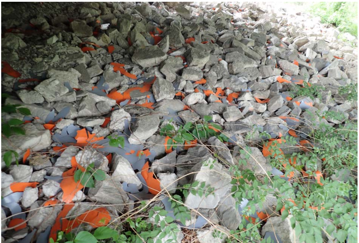
View of paint lying on the ground in span 3.
