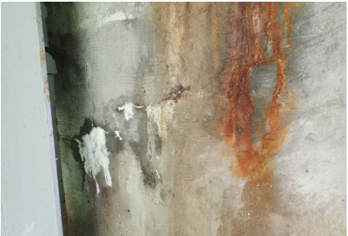
View of minor sized cracking with efflorescence and rust staining in the upstream backwall of abutment 4.
